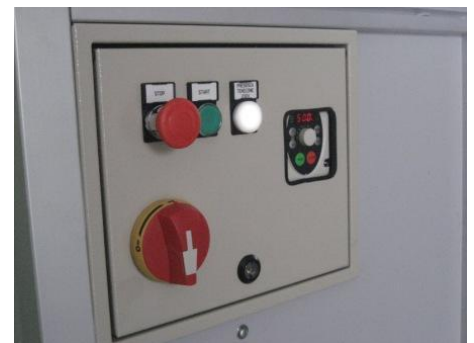
Electric panel with inverter
